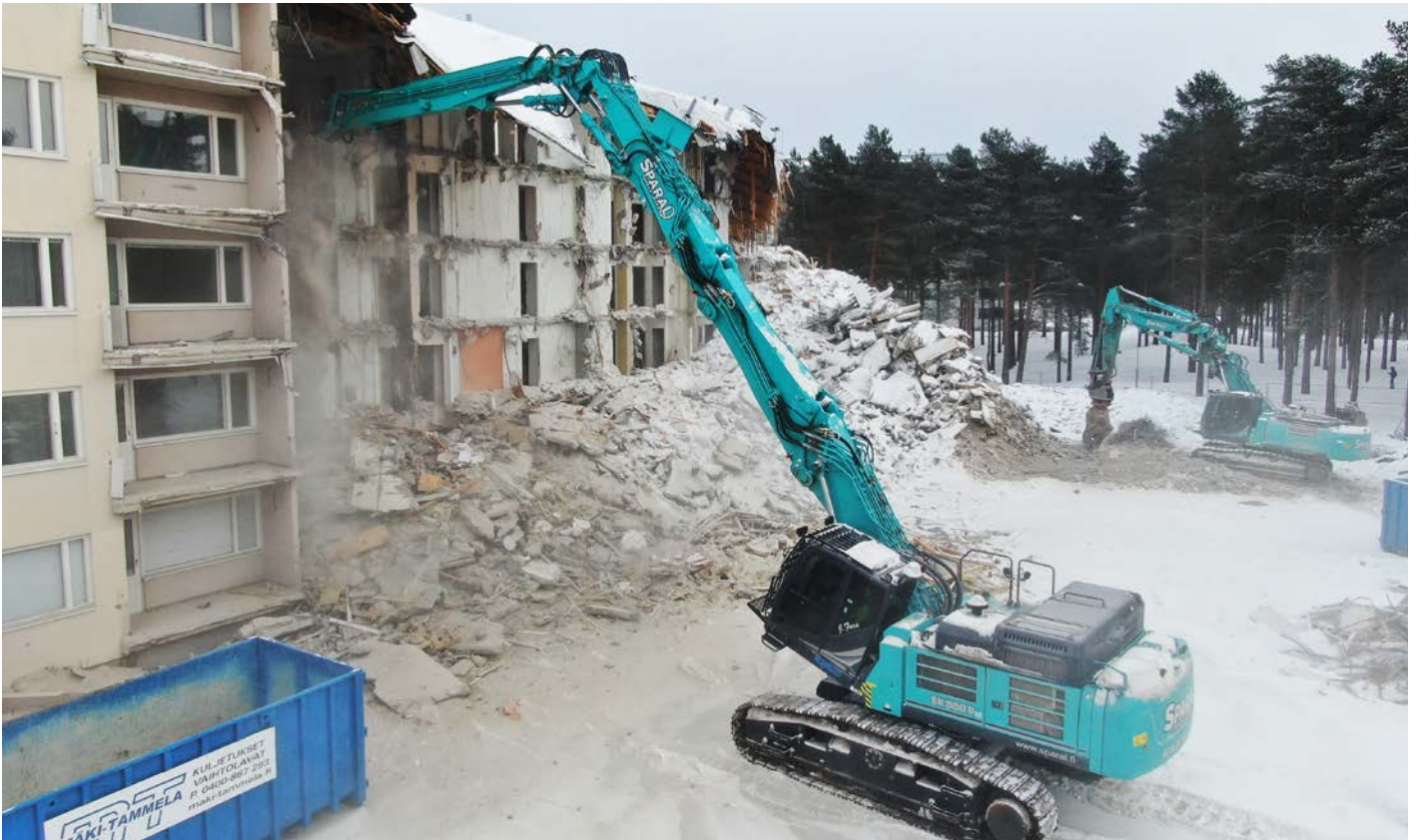
Sparal Oy purchased a Kobelco SK550DLC demolition excavator equipped with a special boom attachment.
